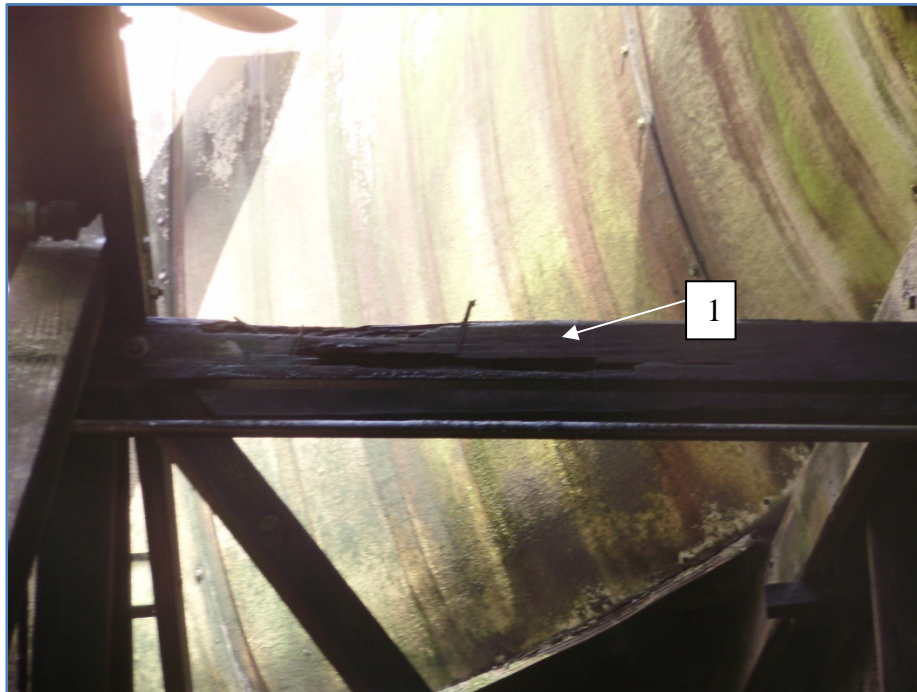
Figure 8: Structural Tie Line- Detail point one refers to a two by four tie line member that has deteriorated from biological rot.
