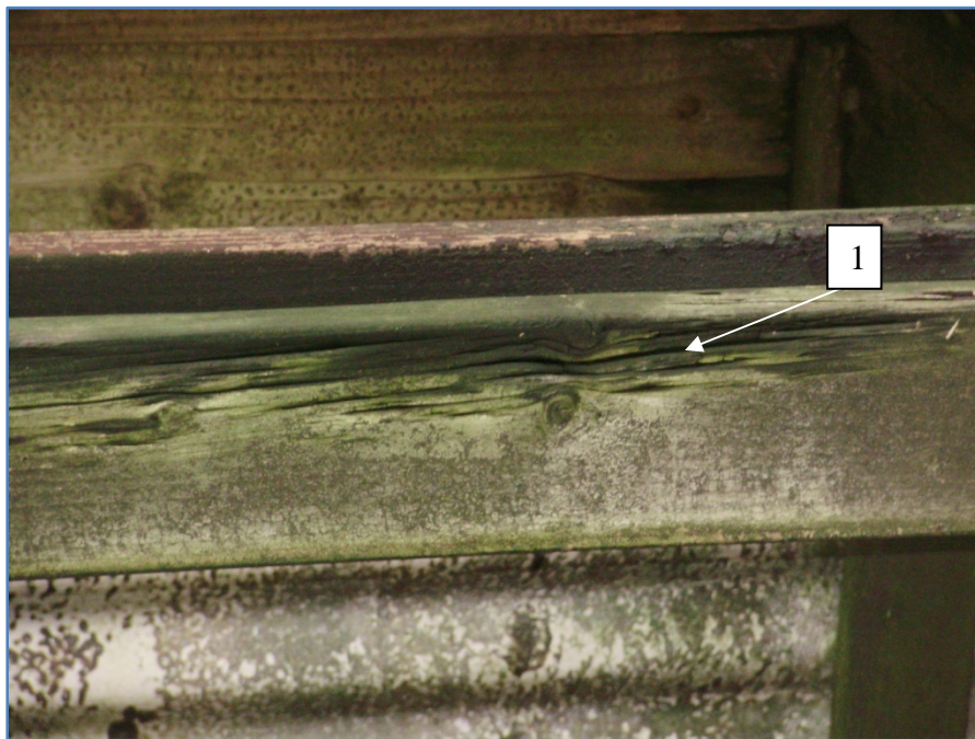
Figure 4: Top Deck- The underside of the cooling tower fan deck, inspection from the plenum area found a few joist members with fungal rot. Detail point one references rot striations in a 2" x 6" joist member in cell number four.
