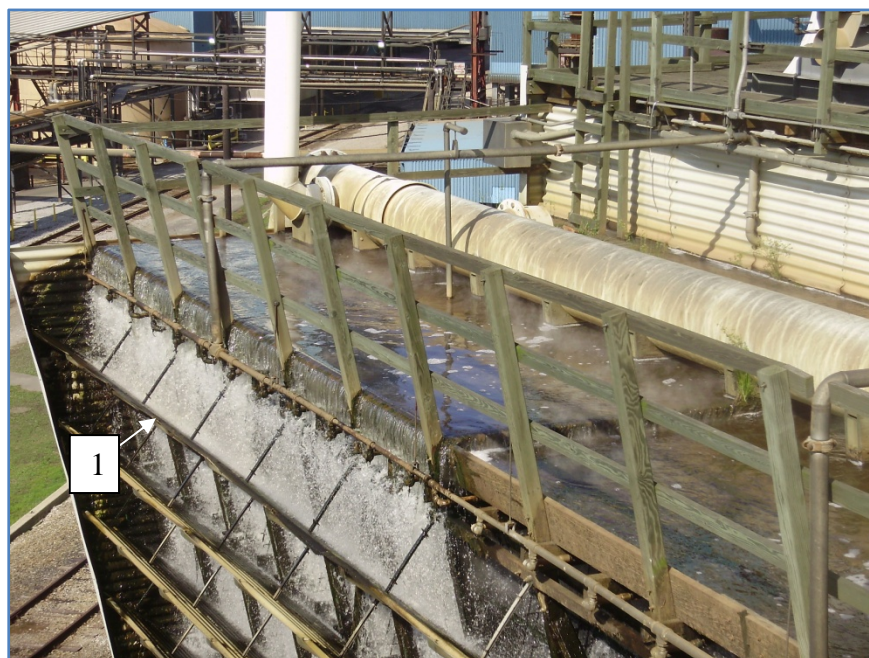
Figure 8: Distribution Deck – two broken flow control valves were found on the tower distribution system. Detail point one refers to the outer curb wall that is engulfed in water. This mass of water restricts airflow through the cooling tower and hinders efficiency.
