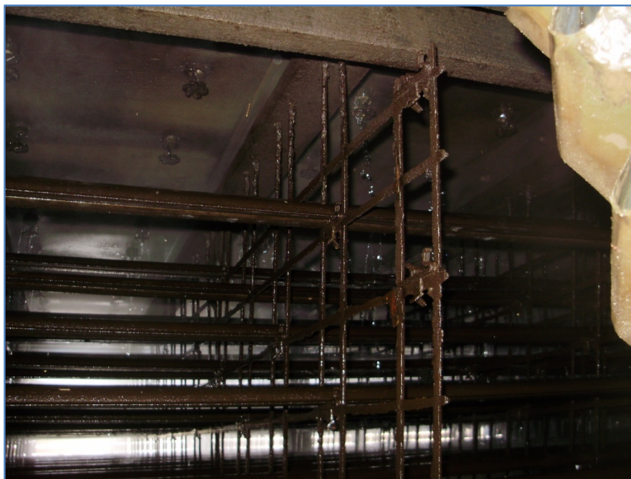
Figure 10: Splash fill material- The fill material was found to be in relatively good condition with no collapsed or significantly damaged sections found at inspection.
