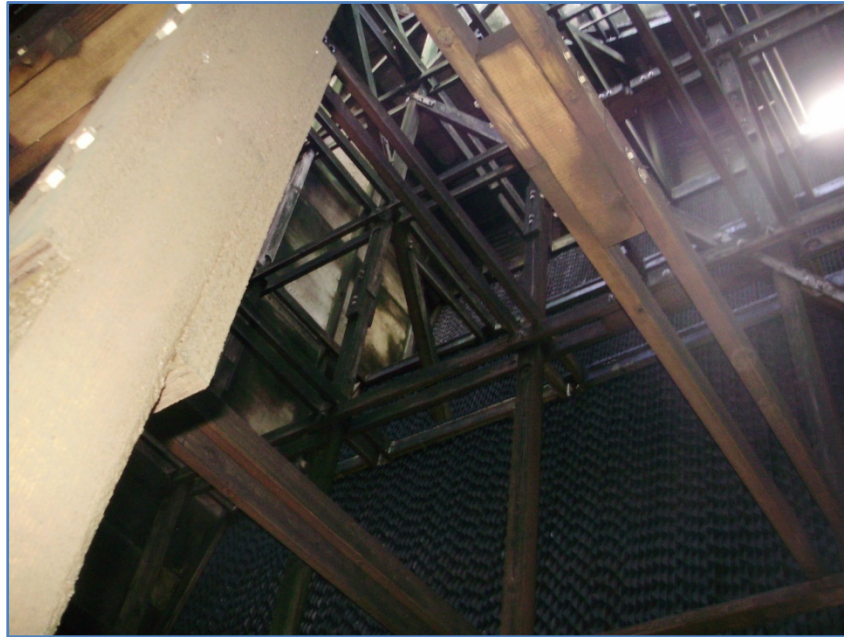
Figure 5: Cell #2 columns -The columns were inspected in upper and lower sections of the plenum and were found to be in good condition.
